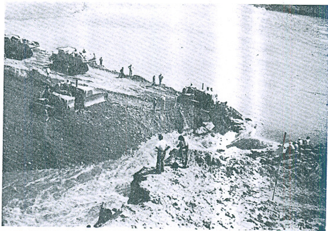
2 Another View of the Closure Operations. The gap is reduced from 58 ft. to 30 ft. The heavy boulders are seen being pushed across by a Dozer. The gravel can be seen immediately on the downstream of the boulders.
