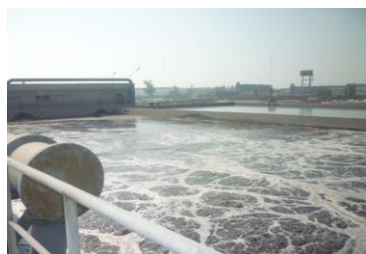
(a) Aeration tank: 1
