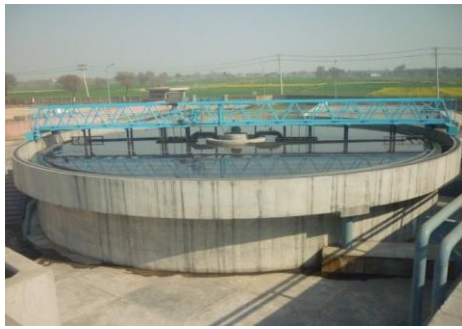
(c) Primary Clarifier
