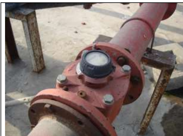
Fig.4 Water Flow meter
