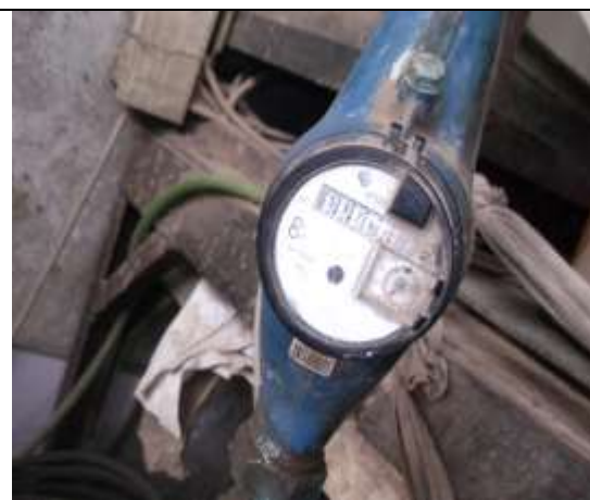
Fig.5 RO water flow meter
