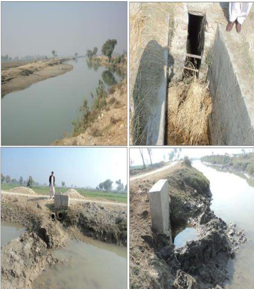
Figure 6: Unner Wah channel (upper right) lost its alignment and x-section; other pictures showing farmers' full authority to divert (or otherwise) water to their outlets.
