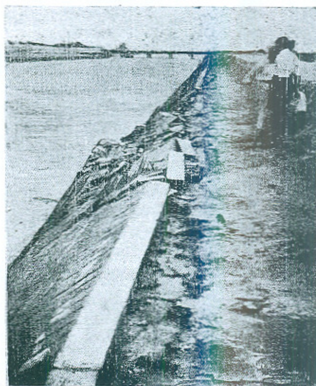
The lining crumbled and slipped.
