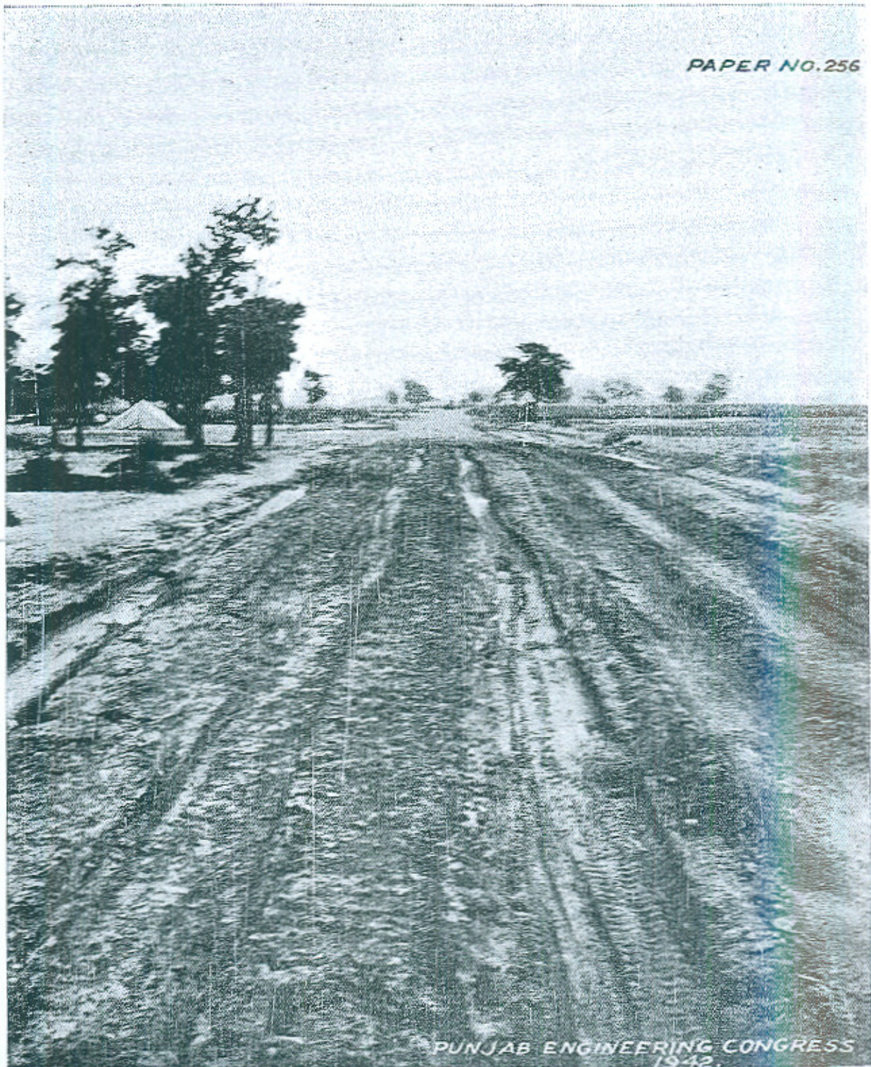
FIG. 2 EXPERIMENT I—KOT LAKHPAT LINK ROAD. SHOWING THE STATE OF THE STABILIZED AND UNSTABILIZED PORTIONS IN THE DRY WEATHER. STABILIZED PORTION CAN BE SEEN IN THE BACKGROUND.
