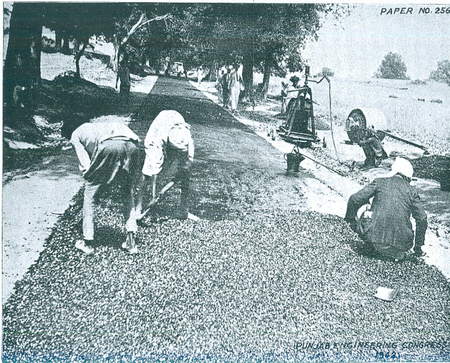
FIG. 7 EXPERIMENT II—HOSHIARPUR-BHARWAIN ROAD. SHOWING THE SURFACING IN PROGRESS. THE TACK COAT CAN BE SEEN IN THE BACKGROUND.
