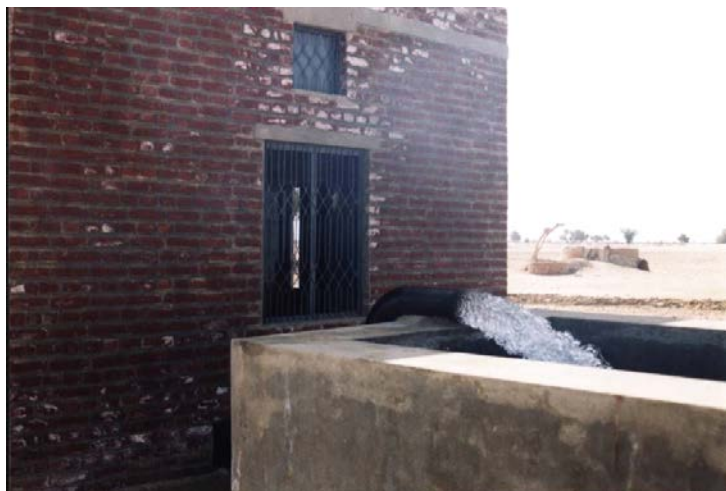
Tubewell Installed by PCRWR
