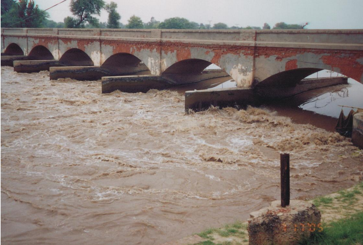
Photo # 3: View of downstream of Fall structure RD 19.11 km Main Canal (LBDC)
