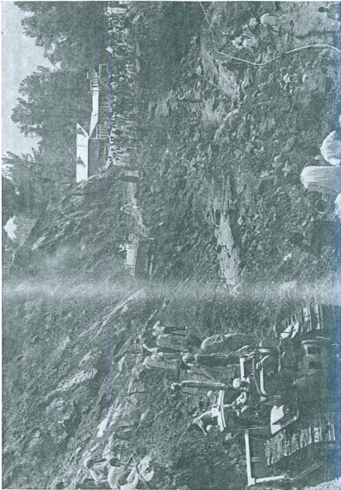
A view of slip affected area in mile 39 showing making of Diversion.
