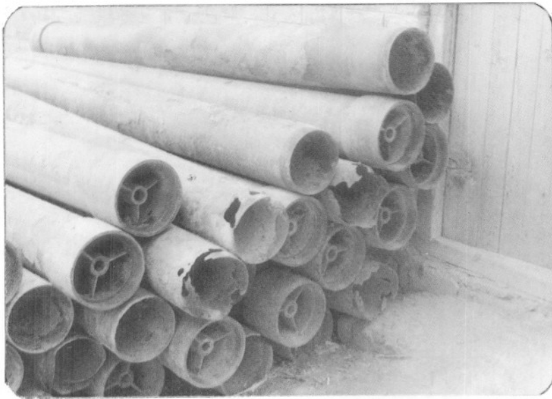
Corroded Coulmn pipes and Shafts (Saline Zone Scarp II)
