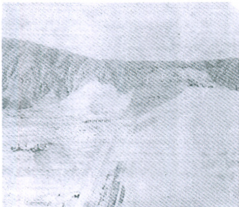
A general view of the downstream face. At peak discharge in August the flow in the Indus reached 11,000 cu m/sec and washed away large sections of the downstream cofferdams around the power station at the foot of the embankment.
