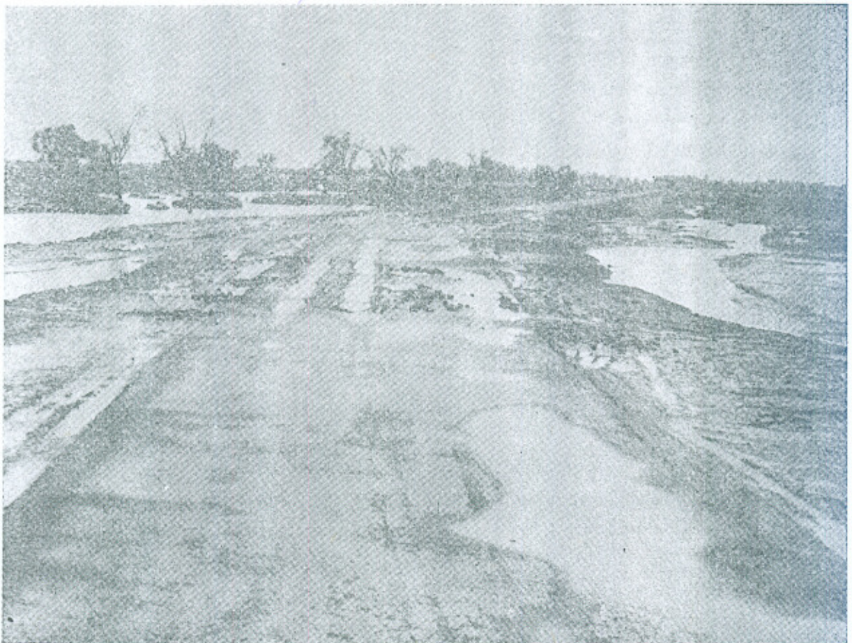
Fig 3. Settled and damaged K hushab Muzaffargarh Road near mile 164 due to waterlogging just near Tail Structure of T. P. Link
