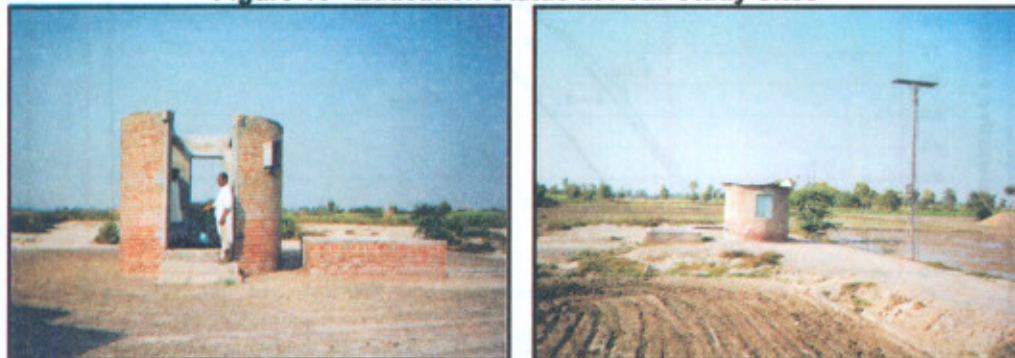
Figure 11 O&M Problems of Sumps at FDP Study Site
