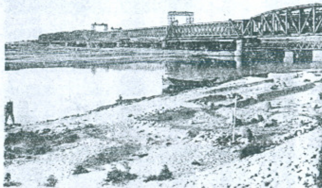
1. GENERAL VIEW OF ERECTION OF SPANS FROM BOTH ENDS OF THE BRIDGE
