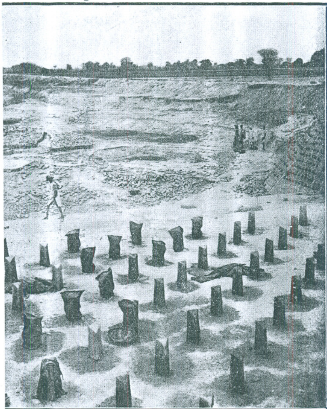
FALL AT R. D. 114000 OF KHADIR BRANCH. REPAIRS IN PROGRESS.
