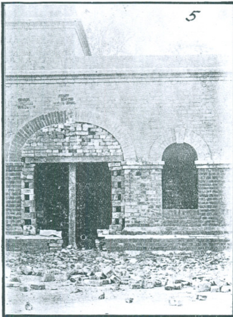
Underpinning of the Verandah pillar and rebuilding the arch up to crown.
